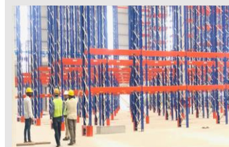
VNA Material storage
